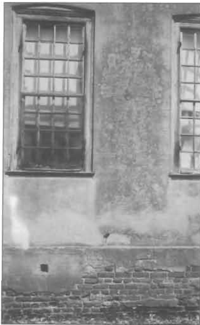
Excessive moisture has damaged not only the stuccoed wall surface, but also the brick substrate.
