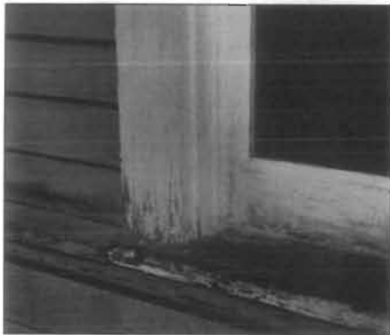
Deterioration of poorly maintained windows usually begins on horizontal surfaces where water collects. Problem areas on this sill are clearly indicated by paint failure due to moisture.
