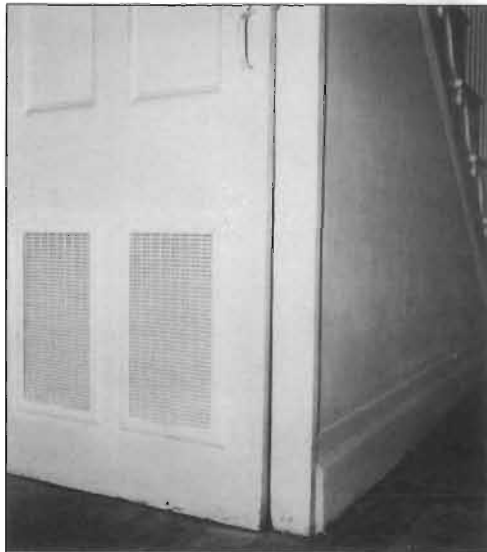
When a late-19th century single-family house was converted to four rental units, the new HVAC system was installed under the central stair. When the door is closed, only the vents indicate its presence.
