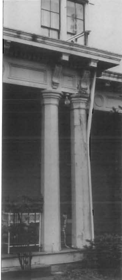
The roof drainage system has been neglected for such a long time that, as a result, the wood cornice and a porch column are both severely deteriorated.
