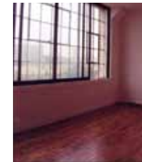
Recommended: [36-38] Original metal windows were retained and made operable during the rehabilitation of this historic mill complex. Installing patio slider doors as interior storm windows was a creative and successful solution to improve the energy efficiency of the existing windows.
